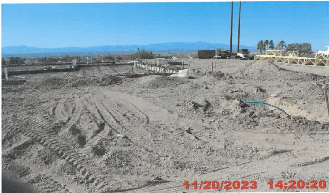
Photograph # 12 Alleged Violation # 1 View of dry, loose, powdery soils, no trackout control device, and active construction activities at 724 Naples Street observed during a follow-up inspection. Photo taken by Andrew Kirk.
