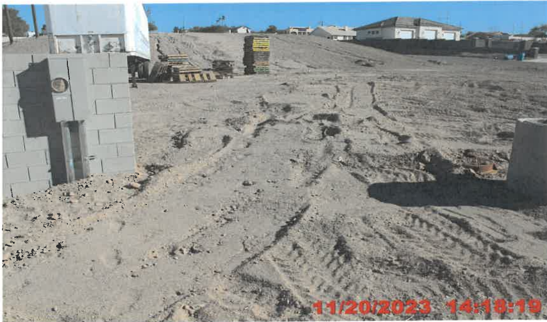
Photograph # 11 Alleged Violation # 1 View of dry, loose, powdery soils and active construction activities at 724 Naples Street observed during a follow-up inspection. Photo taken by Andrew Kirk.
