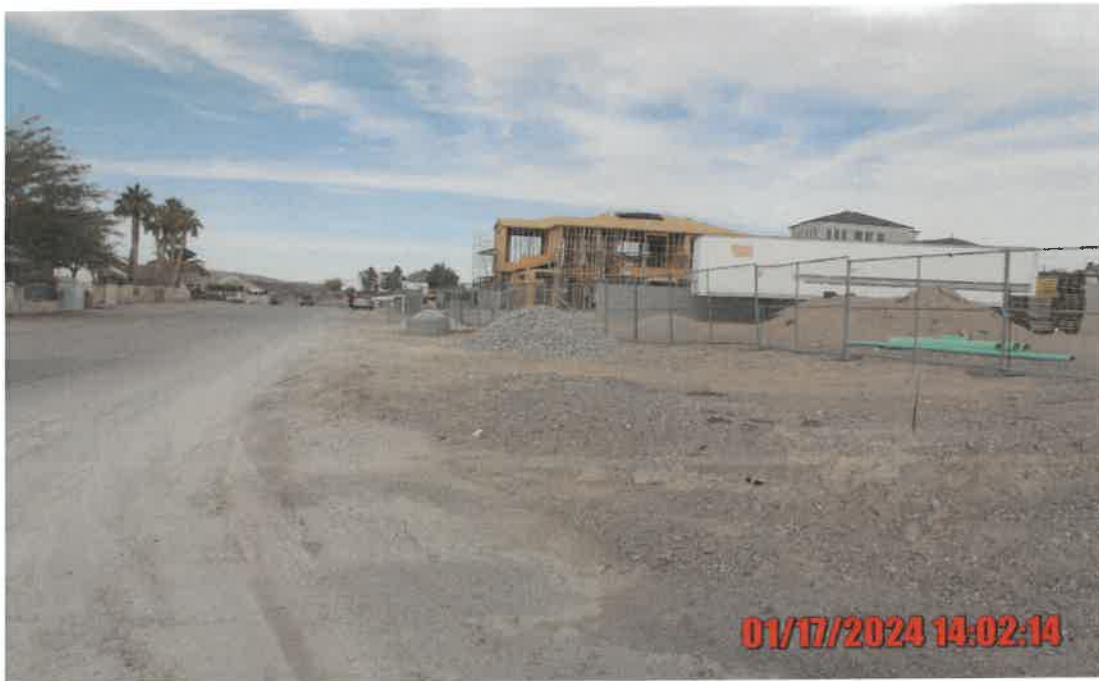
Photograph # 8 Alleged Violation # 1, 2 View looking north at dry, loose and powdery site soils with no available BACM at a project site without a valid dust control operating permit on lot #006, 724 N Naples Street. Photo taken by Senior AQS, Katrinka Byers.
