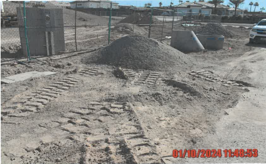
Photograph # 1 Alleged Violation # 1, 2 View looking southeast at dry, loose and powdery site soils with no available BACM at a project site without a valid dust control operating permit on lot #006, 724 N Naples Street. Photo taken by Senior AQS, Katrinka Byers.
